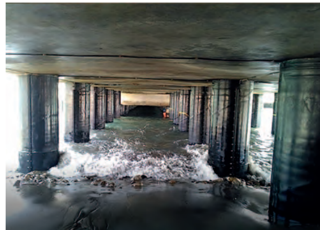
Peru, Port of Talara MarineProtect®-2000 FD 206 piers, DN 1000 (40")
