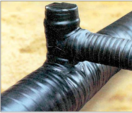
Fig. 6: Typical field of application for type 5.b two-tape system: Coating of weld-on branch line
