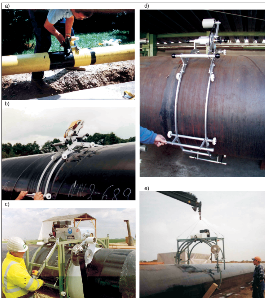
Fig 9: a) Tape wrapping with DENSOMAT 1 hand wrapping machine b) DENSOMAT KGR Junior hand wrapping machine with extension arms c) DENSOMAT 11 motor driven wrapping machine for field joint coating on a 36" pipeline d) DENSOMAT KGR Junior with closed frame e) Easy mounting of DENSOMAT 11 wrapping machine on a 36" pipeline (girth weld insulation)
