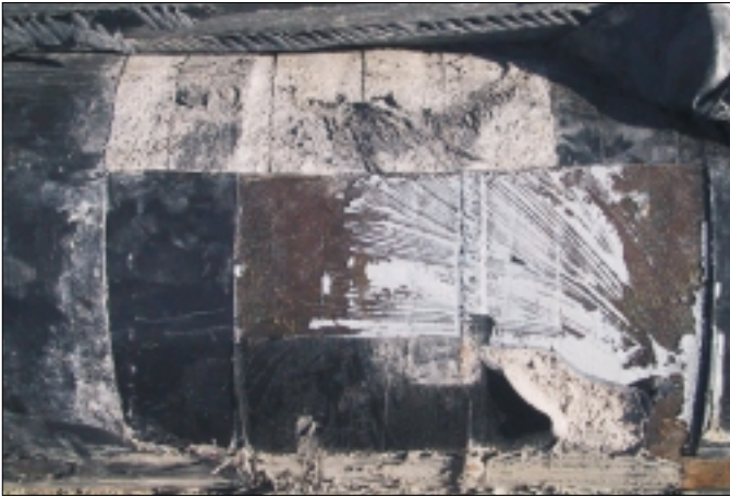
Fig. 4: Partly peeled off welded joint DN 300 with DENSOLEN-System S40
