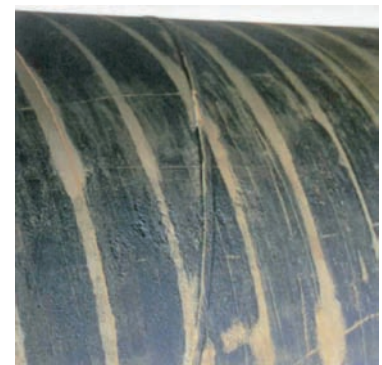
Fig. 4: Spiral corrosion on pipe joint sealing by adhesion only
