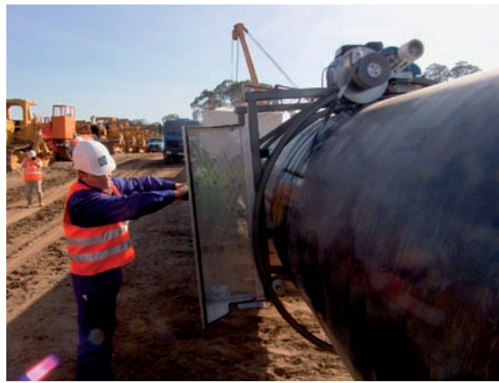
Fig. 13 and 14: Wrapping with engine driven application device-simultaneous application of inner and outer wrap
