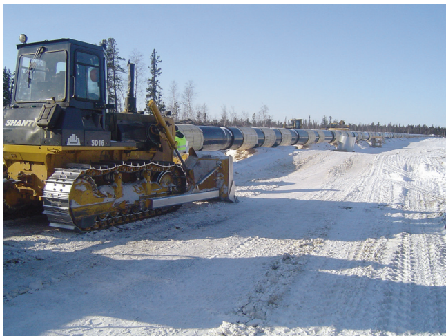
Figure 1. Zapolyarye-Purpe Pipeline Western Siberia.
